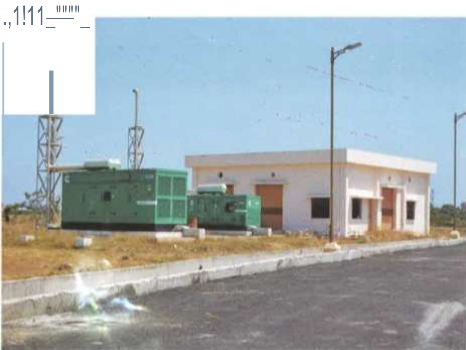
Power Plant Station
